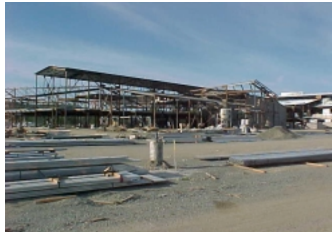
Areas C & D on 06/29/04 - the last areas for steel erection, a phase of work which is now complete.
