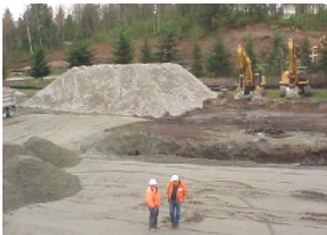
Superintendent George Mason talks with Snohomish County project engineer Ken Miller. In the background is a 1,400 cubic yard pile of crushed concrete recycled from the site.
